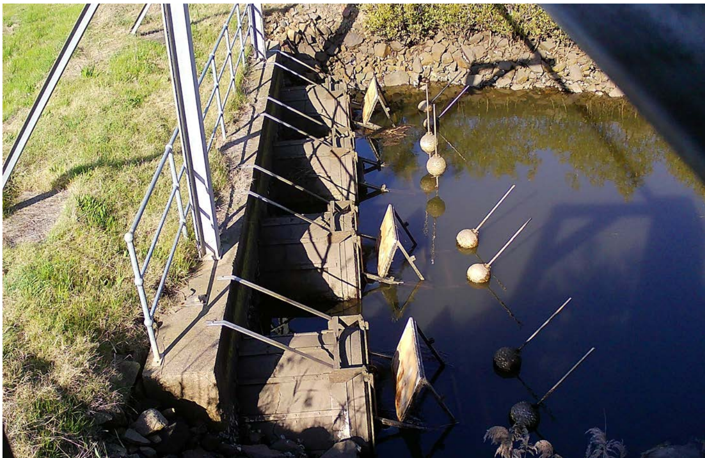
Figure 1.3: SwingGates at Tomago Wetlands.
